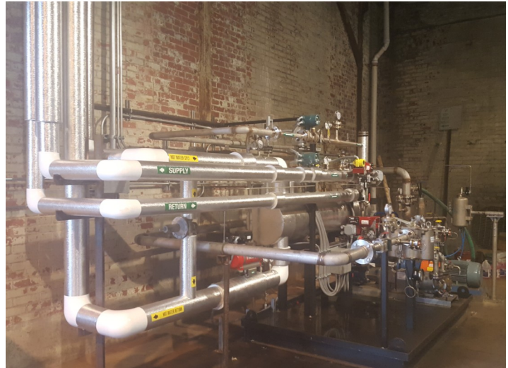
RFO Pump and Heating Skid
